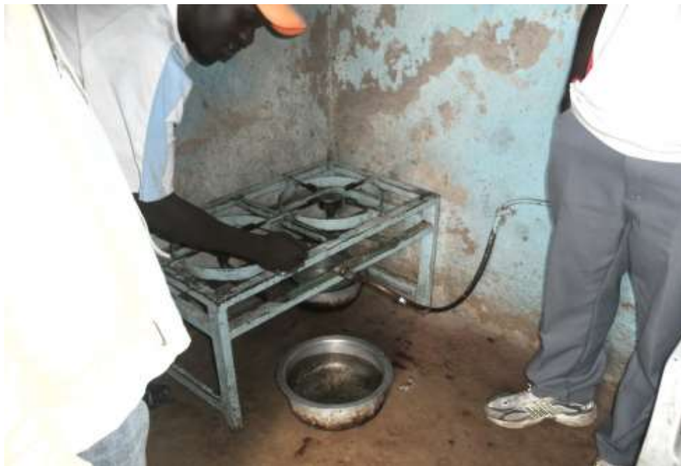
Cooking station at Twaweza Bio-Centre
